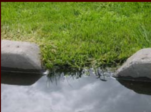
Proper maintenance of the swale inlet can prevent it from looking like this!
