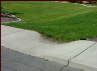
An example of overgrown grass at the inlet of a swale.
