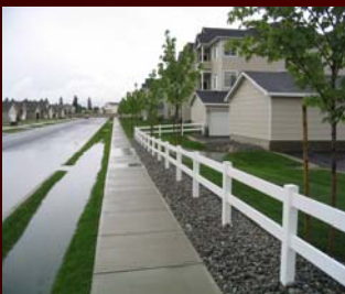
Maintaining your swale will keep it functioning properly and preventing it from looking like this!
